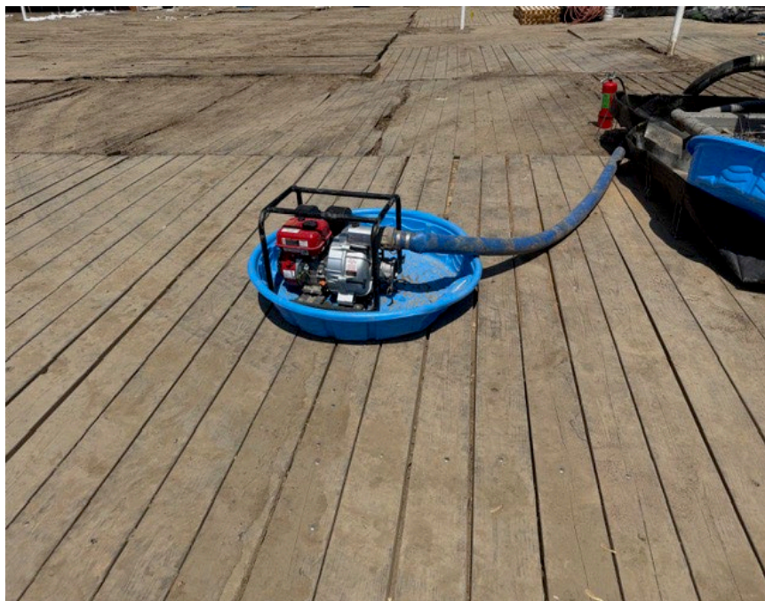
Facing north near MP 2.4, secondary containment utilized
